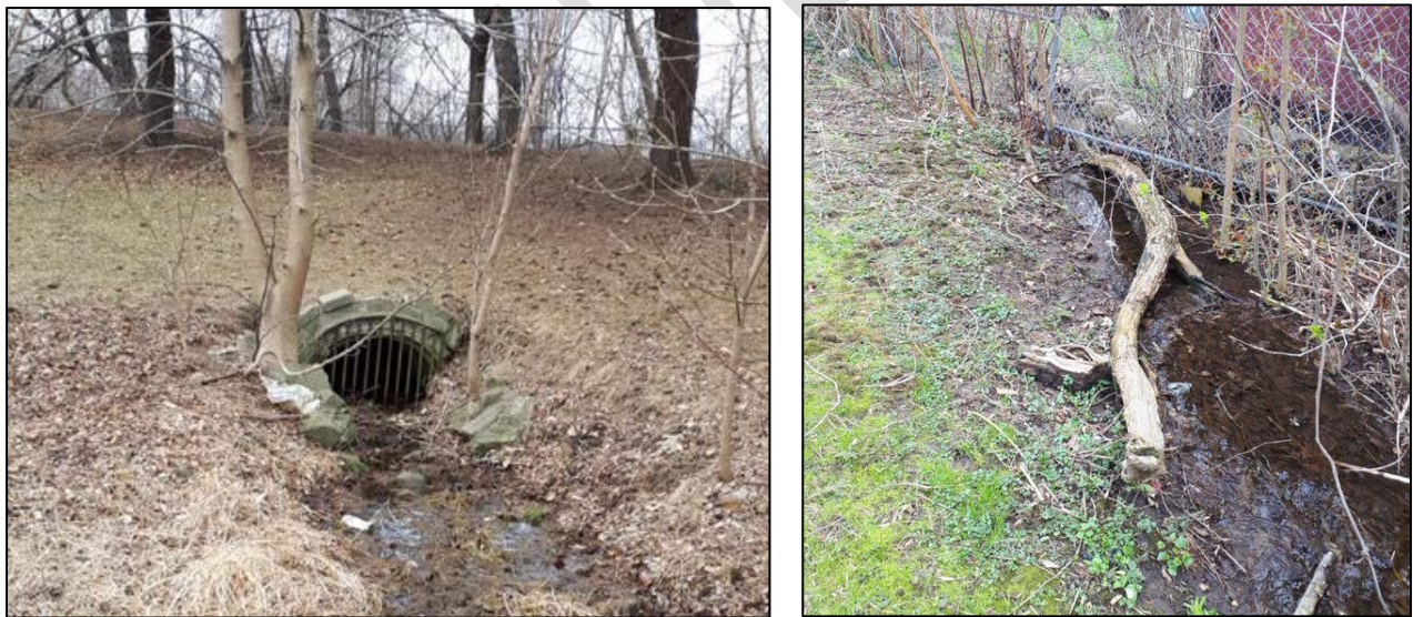
Figure 15: Outflow downstream of Canadian Pacific (CP) rail property (Left), drainage to private property, back yard (Right).
