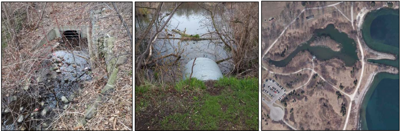
Figure 16: Left to right, Outfall to North Creek at Humber Collage, Outfall to North Creek Wetland, 2019, orthophotography of North Creek Wetland.
